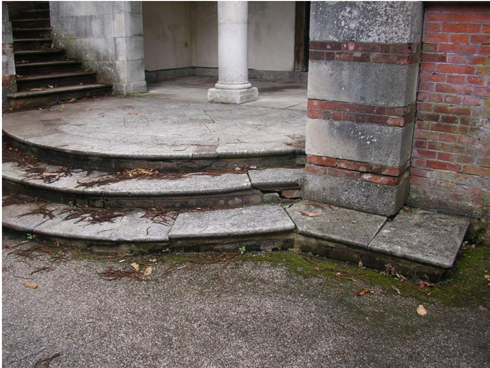
Section 2: cracked staircase at the Belvedere structure which will be repaired as part of the 2015/16 cyclical maintenance programme.
