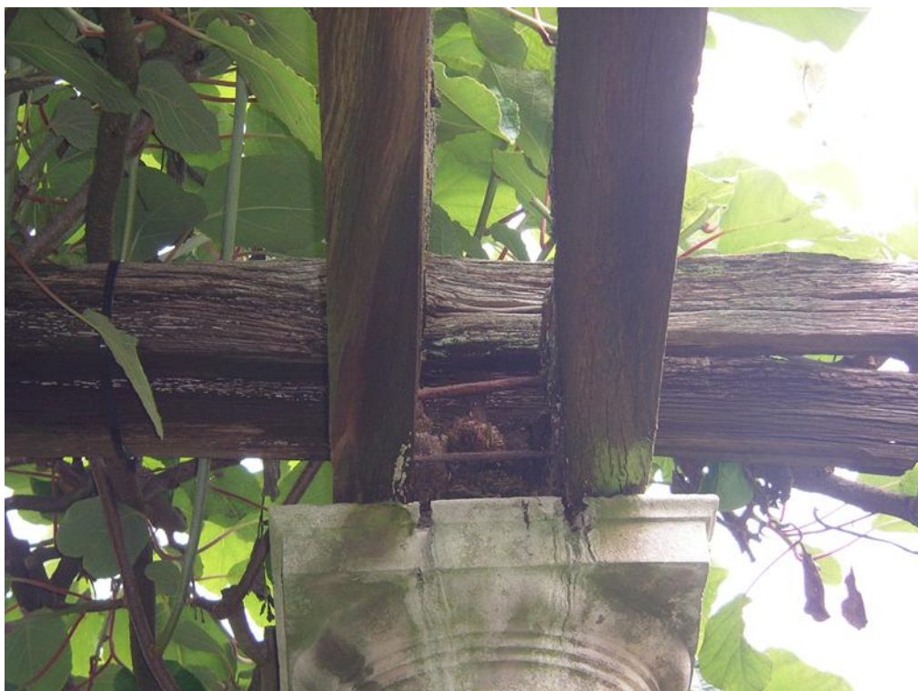
Section 2: showing decayed timbers and acid attack to Portland stone column from oak timbers.
