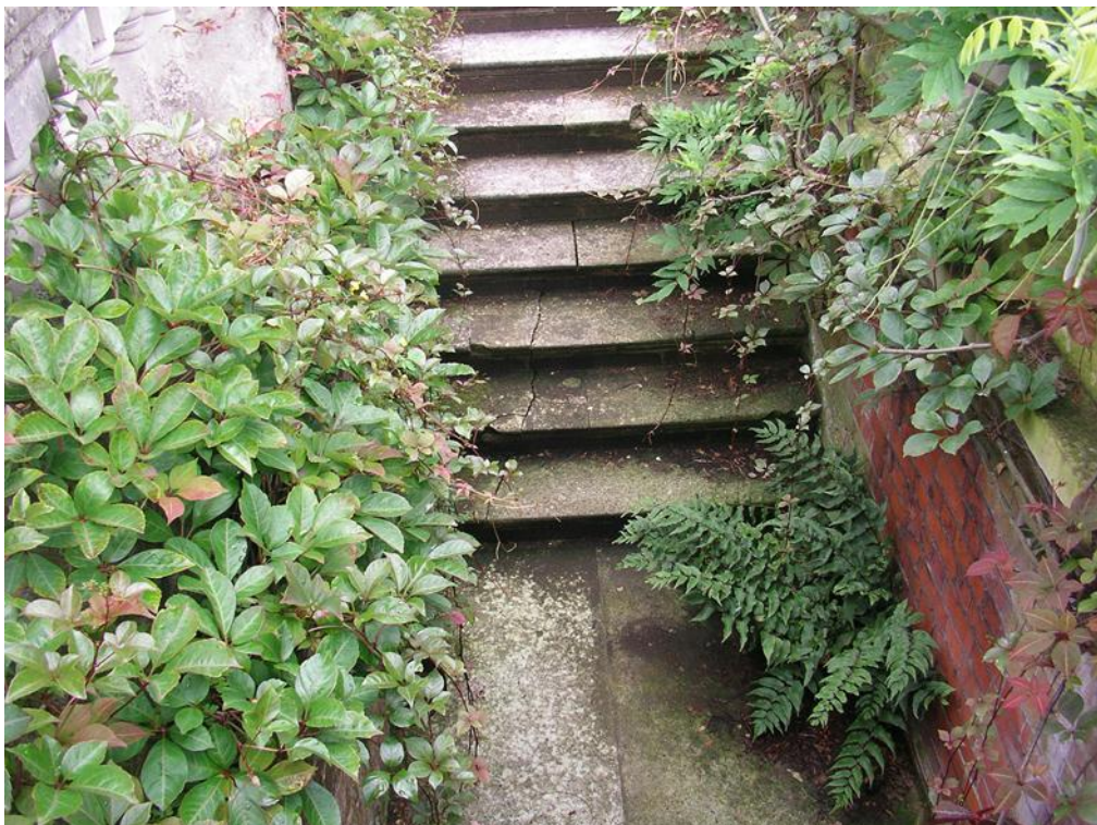
Section 2: one of the minor staircases showing cracked treads.
