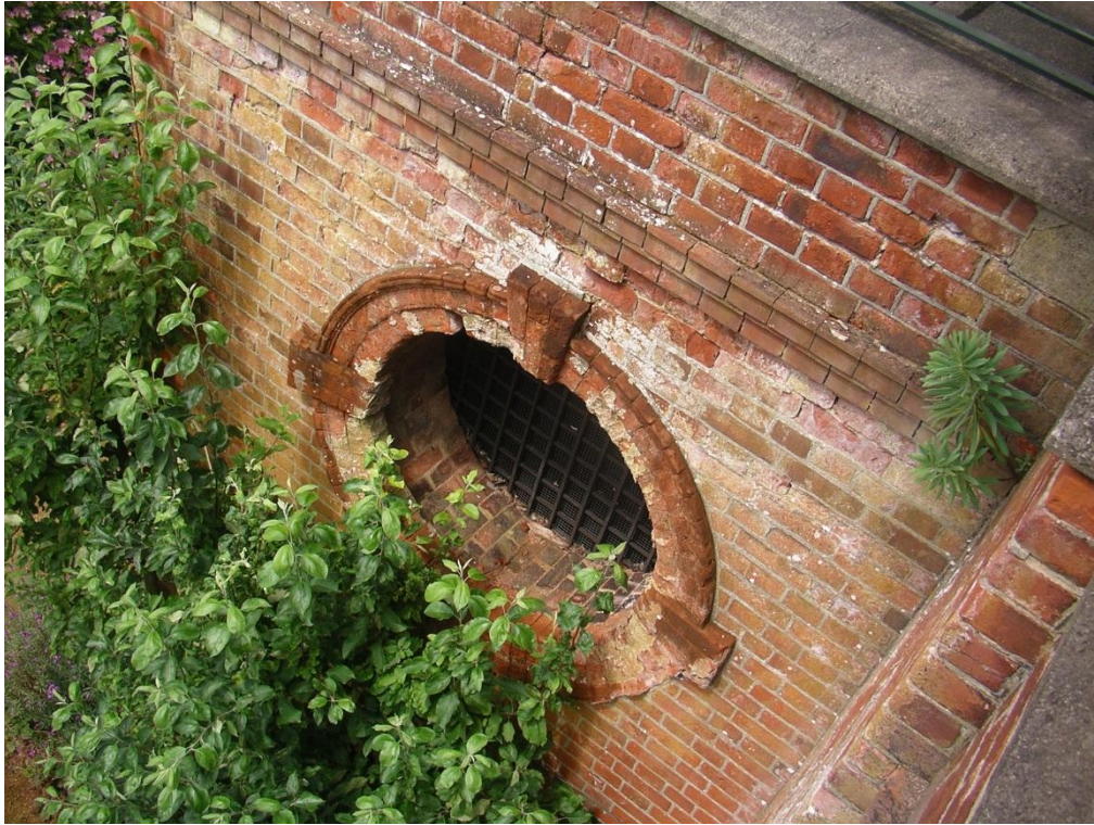
Section 1: brickwork deterioration around a circular window feature and efflorescence below the level of the structural slab to the walkway.
