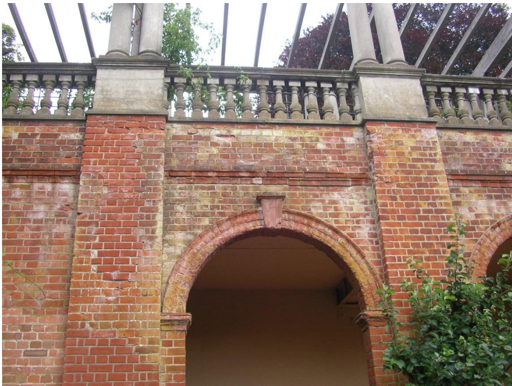
Section 1: Brickwork arcade to lower level walkway showing deterioration due to dampness.
