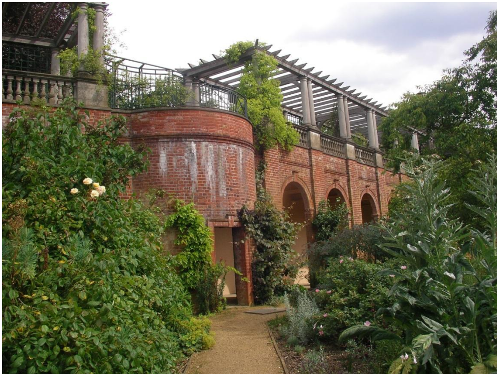
Section 1: The rotunda feature showing unsightly efflorescence.
